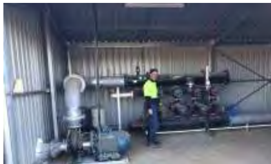
Figure 3.3 Reducing water usage through Sub-Surface Drip Irrigation
