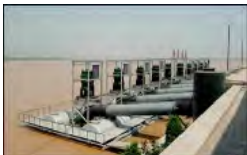
Figure 4.10 Wuwang floating pumping station
