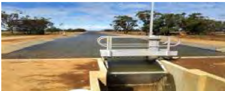
Figure 4.1 Lined channel section with Rubicon control gates
